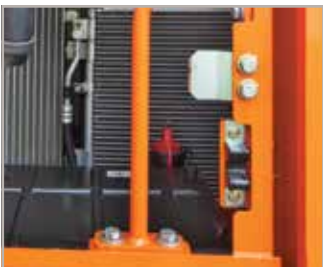
Battery cut-off switch
